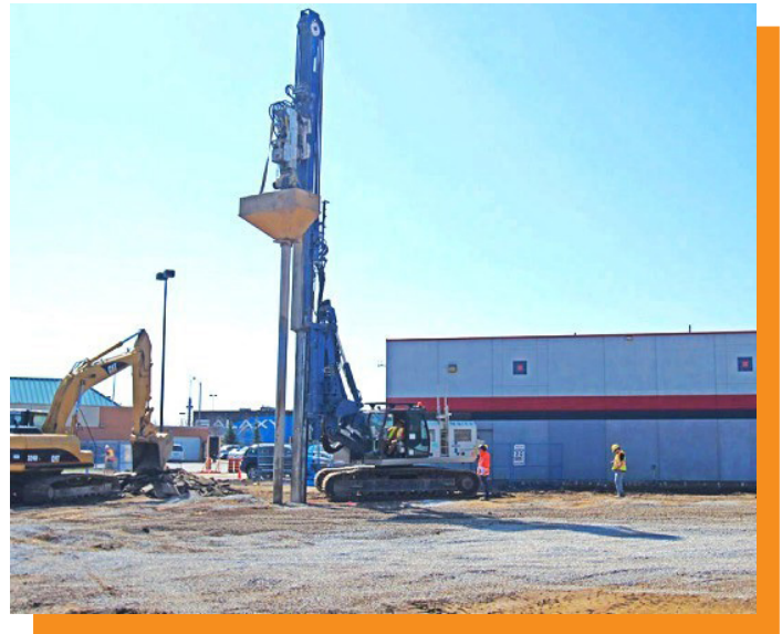
Geopier Impact® work underway for this Walmart addition as part of Walmart's expansion into groceries in Ontario
