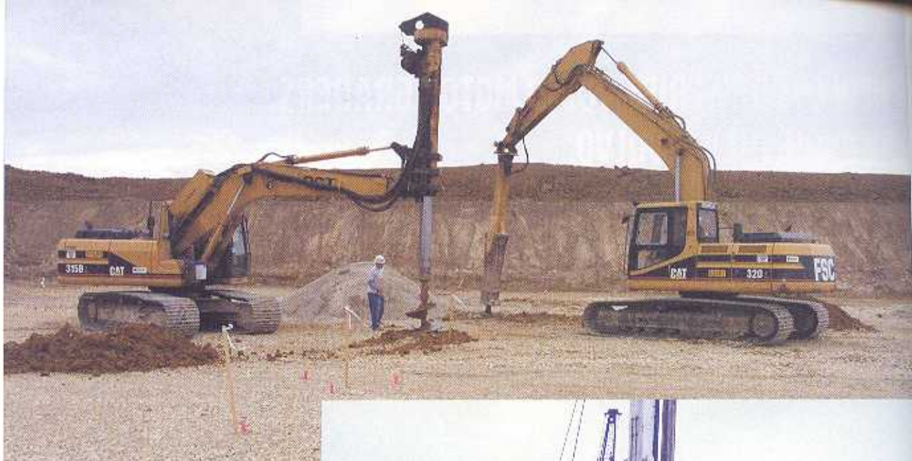
Above: Two of the key attachments in Geopier installation are the drill and the rammer on a Caterpillar 315B and 320, respectively.
