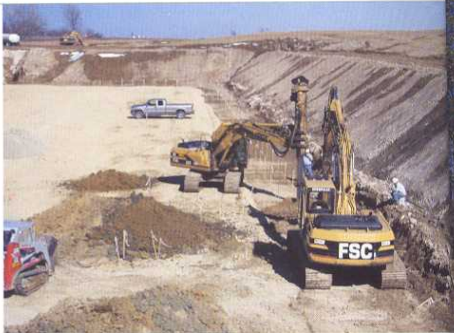
Geopier elements are installed for a retaining wall at Jordan Creek Town Center in West Des Moines.
