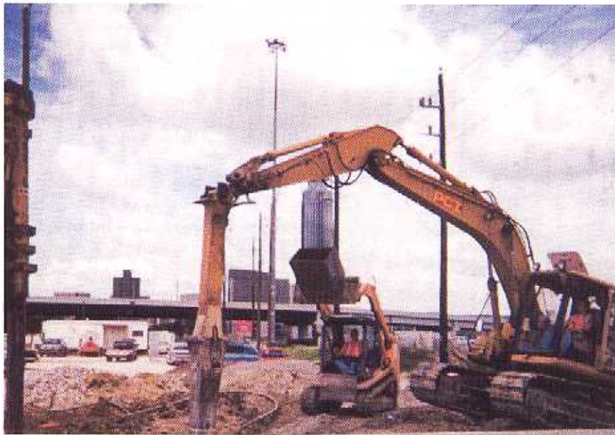
A hydraulic tamper rams aggregate at 1.3 million foot pounds energy per minute to form a Geopier element as a skid loader with custom bucket brings aggregate to shaft. Photo by Tommy Williamson.
