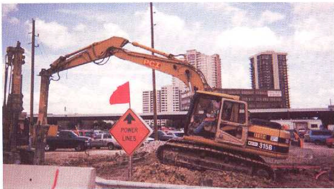
Working around utilities challenges both Geopier installers, Peterson Contractors Inc. (PCI), and Champagne-Webber, general contractor for Section 15 of Houston's Westpark Tollway. Photo by Tommy Williamson.
