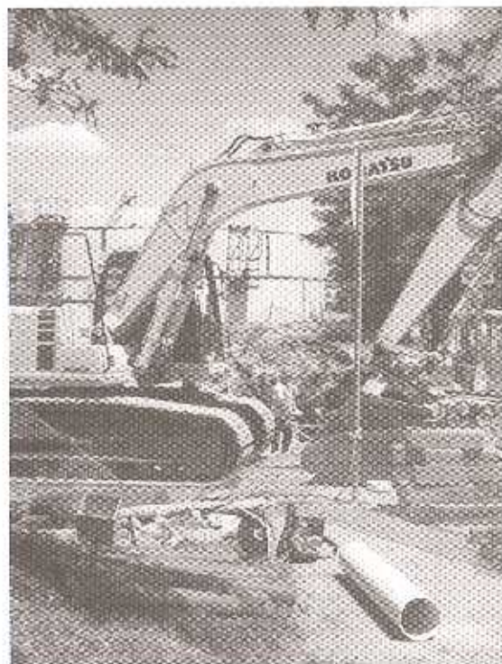
District Cooling St. Paul (DCSP) Inc., an affiliate company of District Energy St. Paul (DESP), currently is expanding the energy system operated by DCSP.
