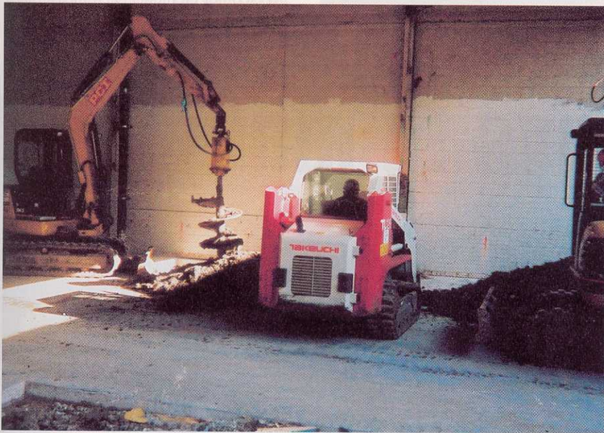
Above: A rented Cat to the left is drilling a hole, while a rented Takeuchi TL 126 skid-loader delivers stone to a previously drilled hole. The skid-loader is equipped with a specially designed bucket to deliver a 12-inch lift of stone dropped down the hole, prior to tamping.
