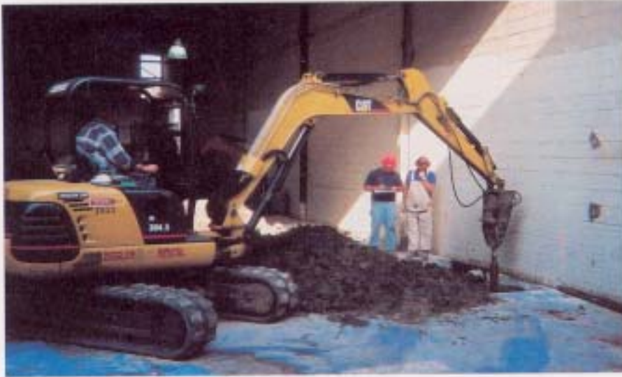
A tamper mounted on a rented Cat 304.5 rubber tracked hoe compacts the lift of stone to form the Geopier element.
