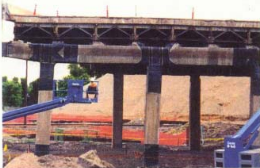
Carbon-fiber reinforcements improved performance of bridge bents subjected to the University of Utah's earthquake study.
