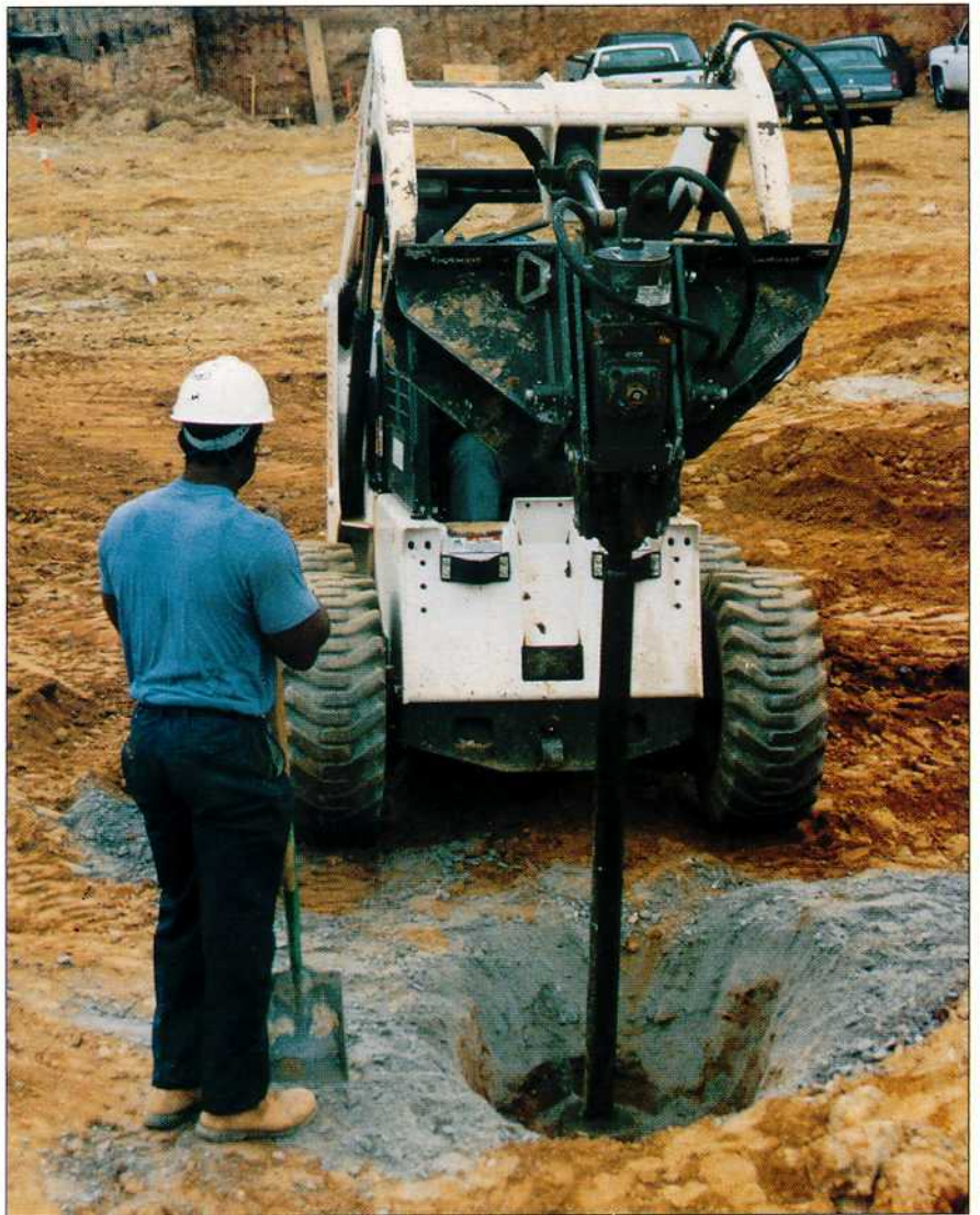
A SMALL GEOPIER-INSTALLING SYSTEM INVOLVES A SKID LOADER WITH A MODIFIED HYDRAULIC BREAKER AND SPECIAL GEOPIER TAMPER TO COMPACT THE AGGREGATE.
