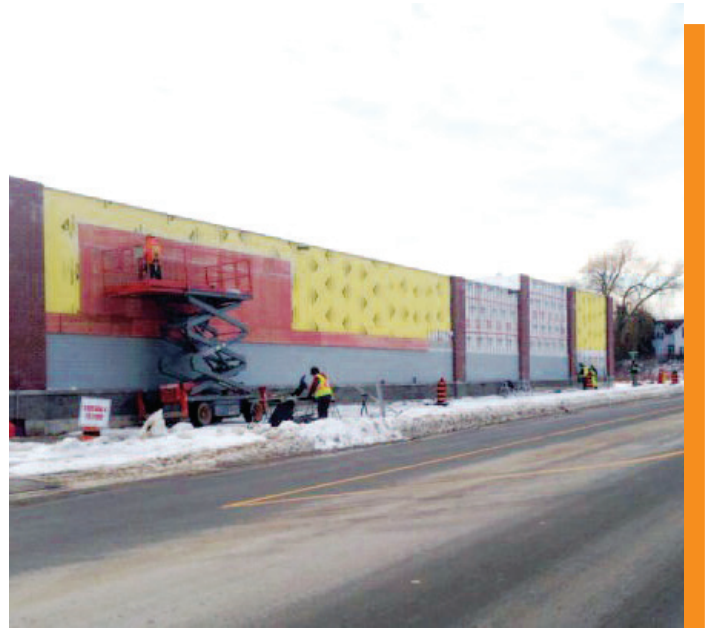
Utilizing Geopier's GP3® system allowed for winter construction to take place on this important project
